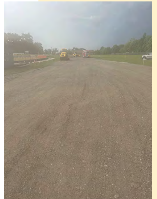
Temporary hauling roads will help truck traffic access the site and minimize soil erosion.
