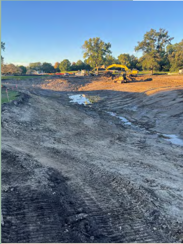
Heavy earth excavation of the Par 3 Storage Facility continued into the new ponds.
