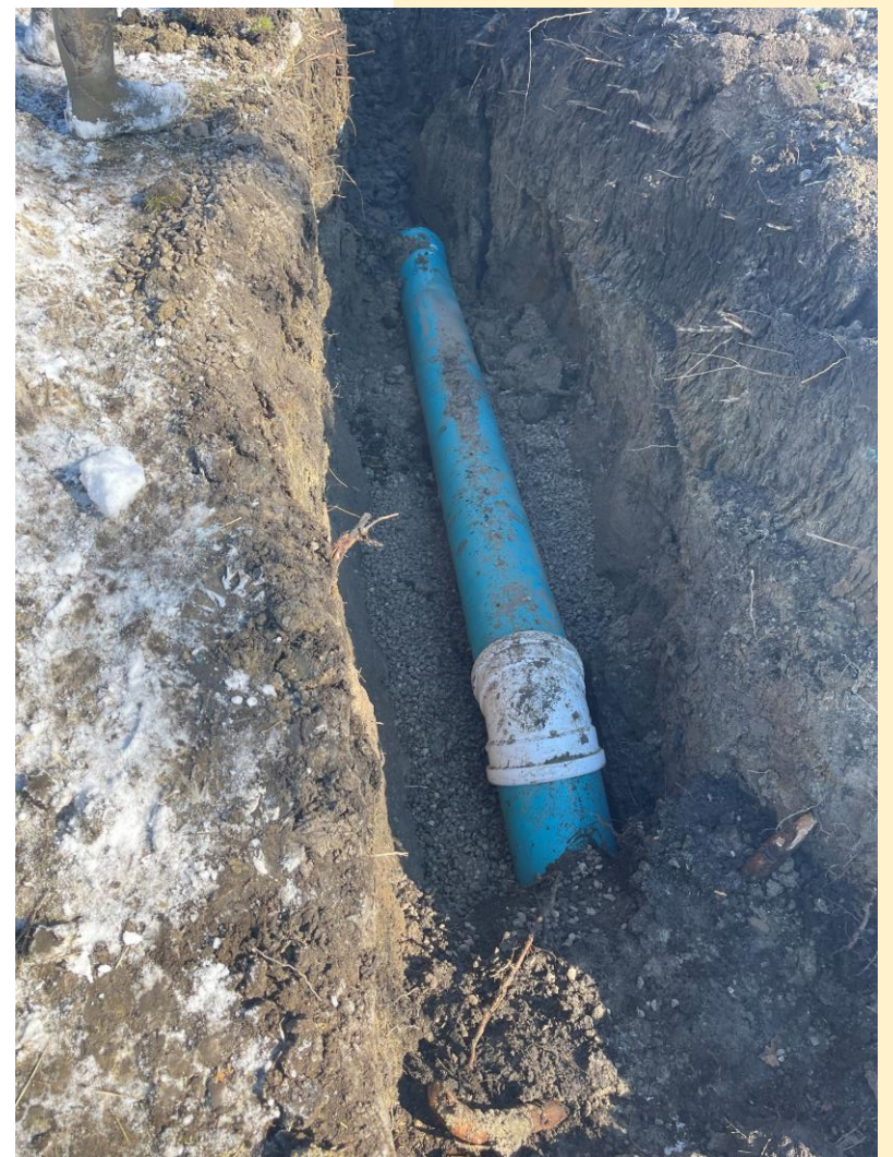
DiMeo rerouted the Winnetka Golf Club sanitary service under the Par 3 Course
