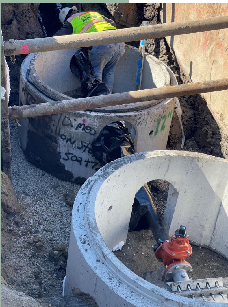
DiMeo works to install a new 4" water service to the Duke Childs Complex
